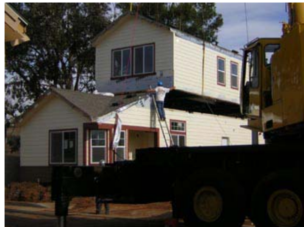
Workers attach the second level of a manufactured home in Brotherton Square.
